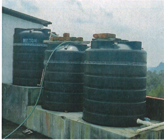
College Building water tank
